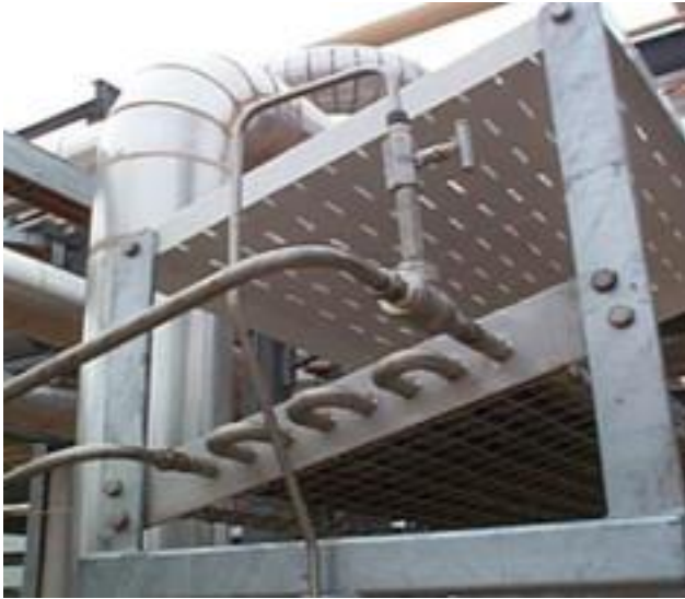
Figure 2. Natural Convection Air Cooler with a Solar Shade
