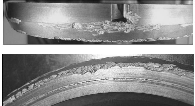
Figure 1. Electro corrosion on an \alpha -SiC rotating seal face, used in an European reactor feed pump seal
