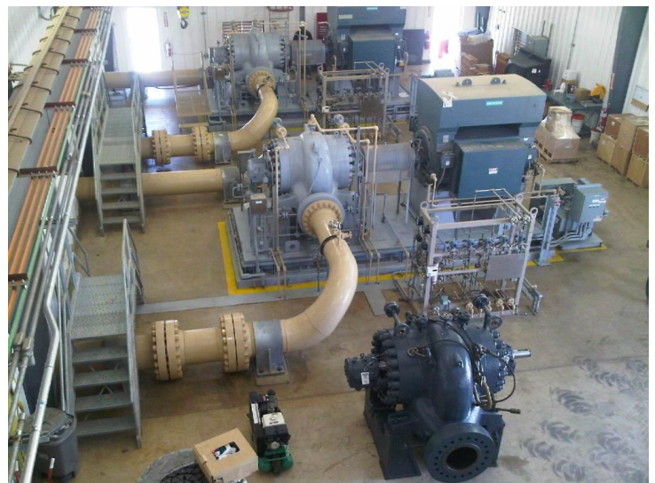
Figure 22. Pump Station (Courtesy Kinder Morgan)
