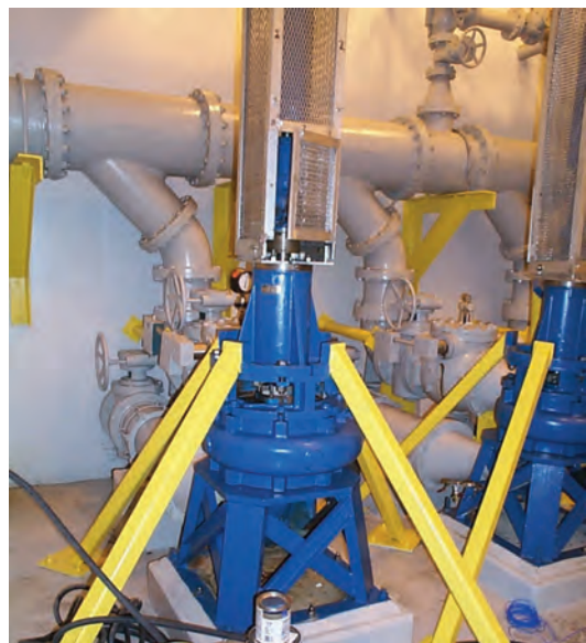
Figure 56. Photo of the Pump Assembly with the Braces.
