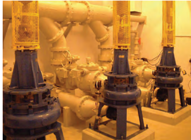
Figure 41. Sewage Pumps Mounted on Fabricated Stands.
