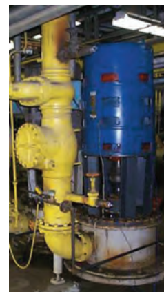
Figure 29. Vertical Turbine Canned Pump Motor Supported on the Stand.
