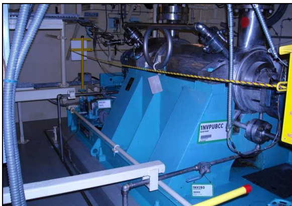
Figure 2. Photo of the 1B NV Pump
