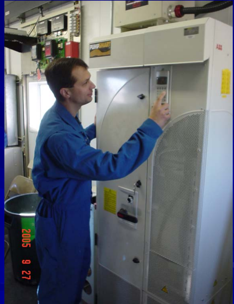
VFD Configured for Dual Speed Operation
