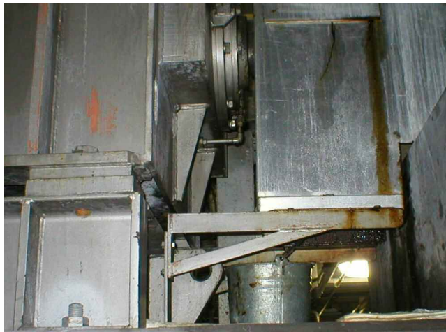
Figure 21. Gearbox at a Newsprint Mill, Leaking Oil Prior to Installation of Magnetic Bearing Isolator. (Courtesy Industrial Packing Company)
