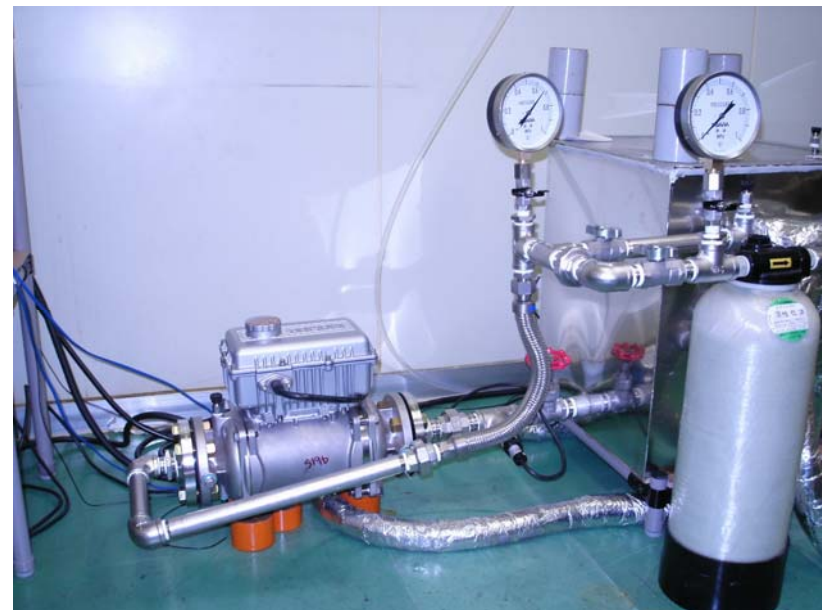
Pump running test
