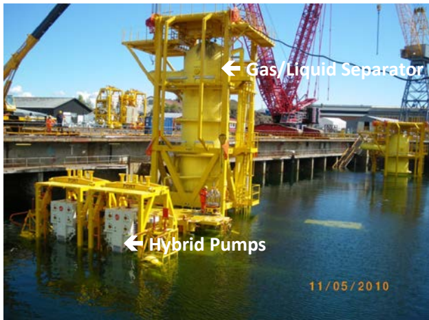
Figure 14. SSU during Shallow Water Functional Test (Courtesy of Pazflor Project)
