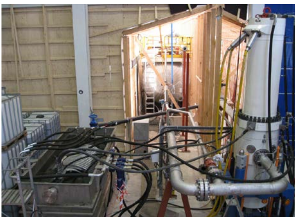
Figure 4. Pump Performance Test (Courtesy of Pazflor Project)
