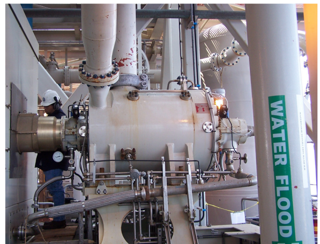
Figure 18: Application 1 Installed Pump
