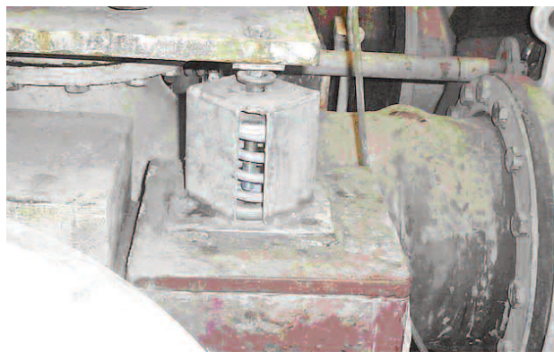
Figure 9. Replacement Spring Isolator and Wide Arch Flexible Coupling.
