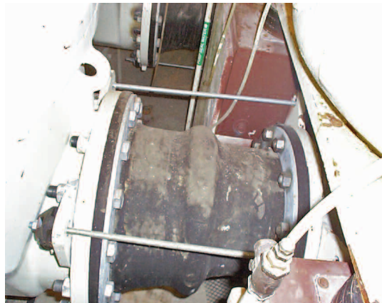
Figure 10. Picture of Original Flexible Coupling.
