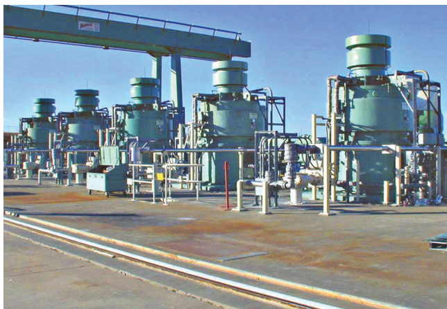
Figure 1. Installation at Power Plant.
