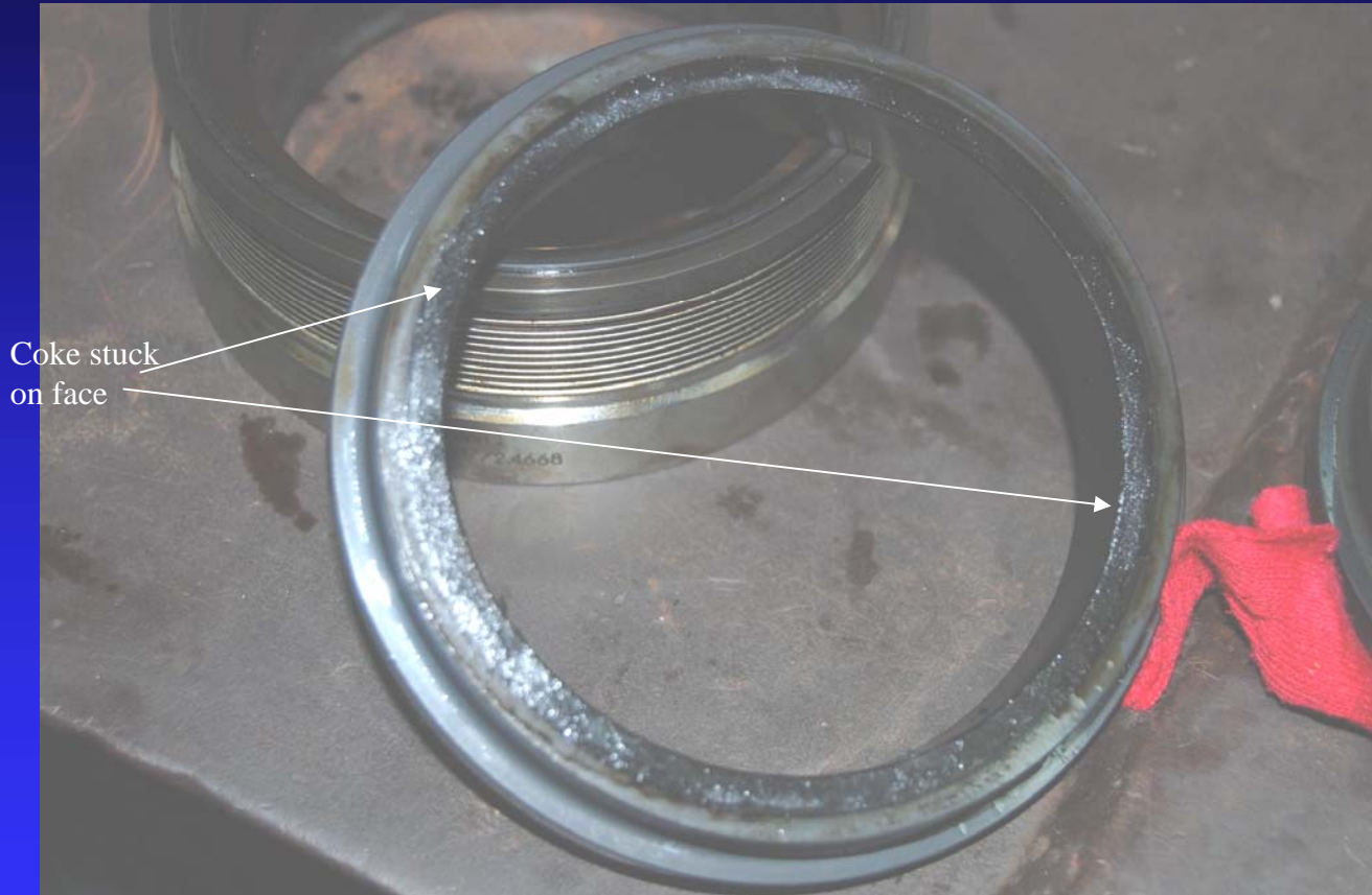
Picture 2: West Feed Pump Interstage End – Inner Seal Face (Stationary)
