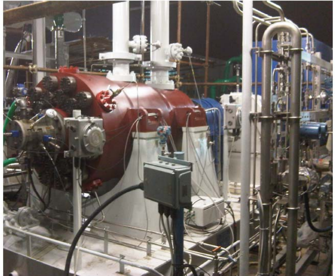
Offshore CO2 reinjection in Brazil, 2010
