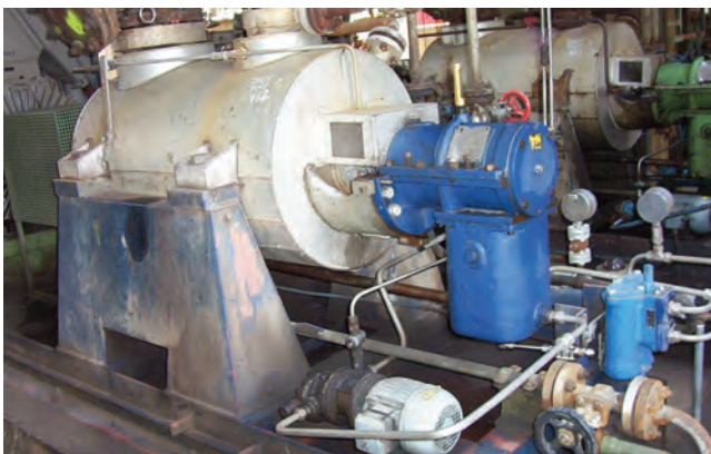
Figure 15. Barrel Pump at Site after Retrofit.
