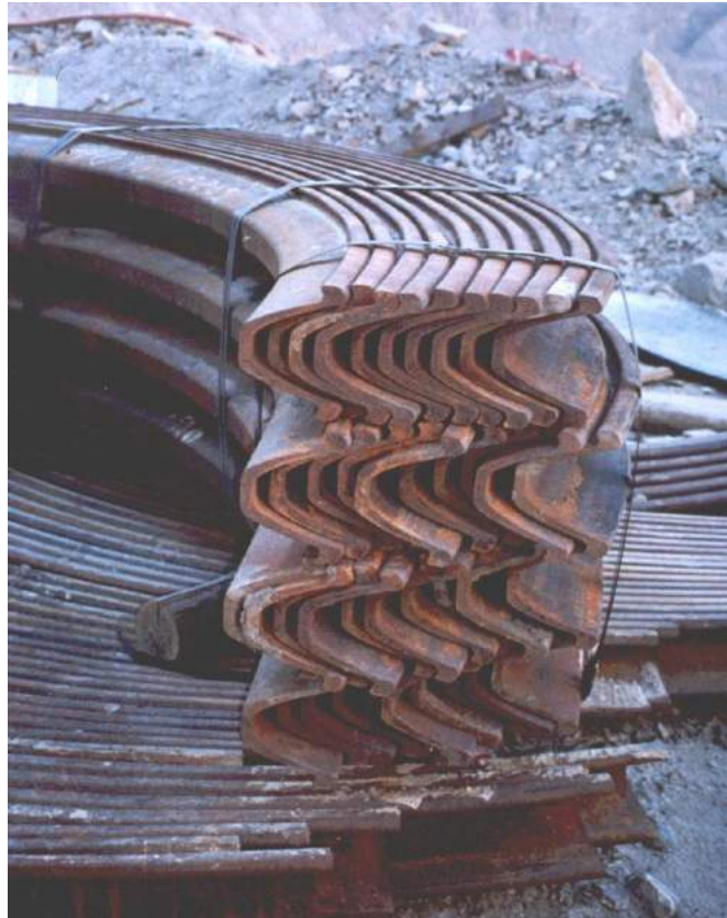
Figure 13 Top hat section steel sets delivered to site ready to be transported underground.
