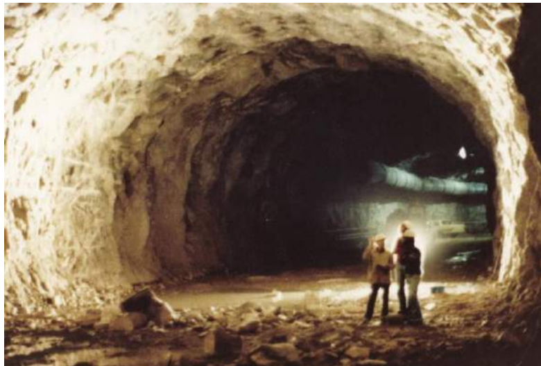
Figure 21: Top heading of the 12 m span, 18 m high tailrace tunnel for the Rio Grande Pumped Storage Project.
