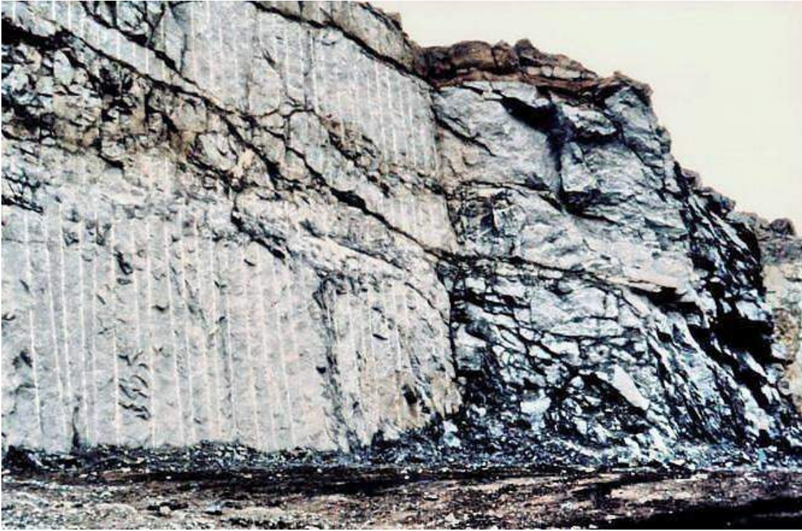
Figure 6: Comparison between the results achieved using controlled blasting (on the left) and normal bulk blasting for a surface excavation in gneiss.
