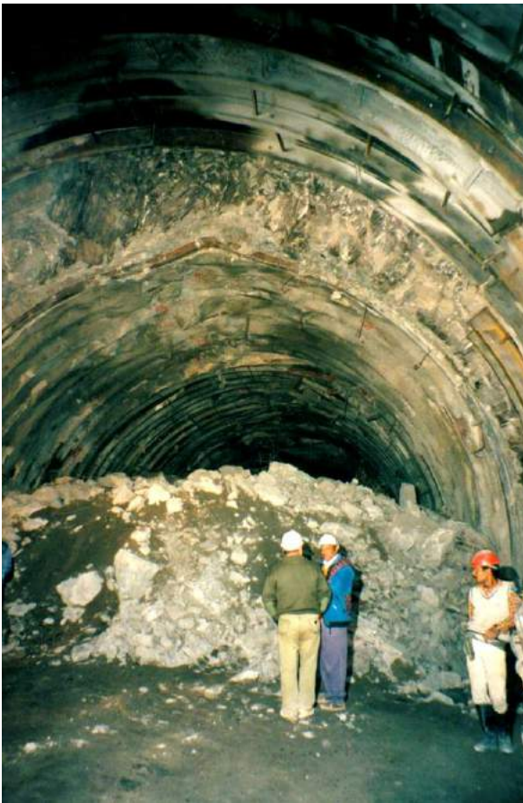
Figure 24: Large displacements in the top heading of the headrace tunnel of the Nathpa Jhakri Hydroelectric project. These displacements are the result of deteriorating rock mass quality when tunnelling through a fault zone.
