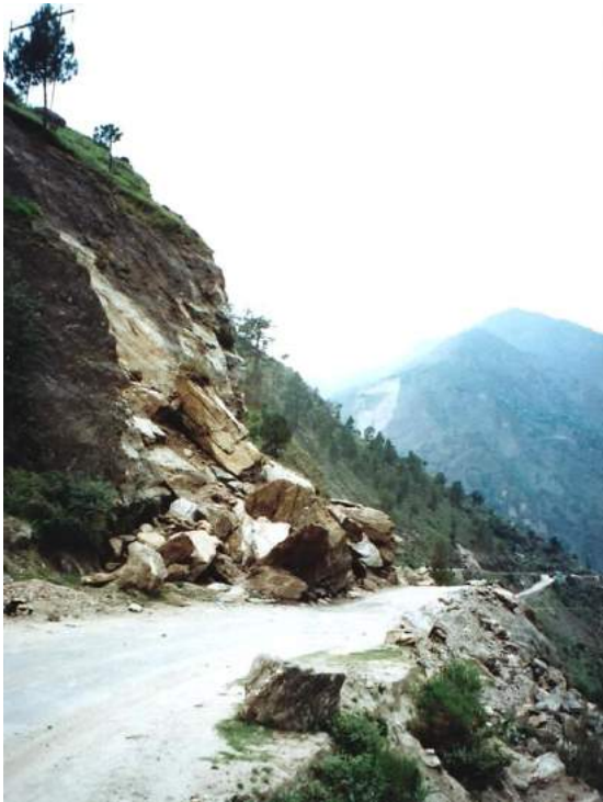
Figure 3: A rock slide on a road caused by the undercutting of sheet joints in a granite slope. In hard rocks such as granite, failure can occur very suddenly if the factor of safety of the slope is close to 1. A rise in groundwater levels during a heavy storm or ice jacking in winter may be sufficient to induce failure.
