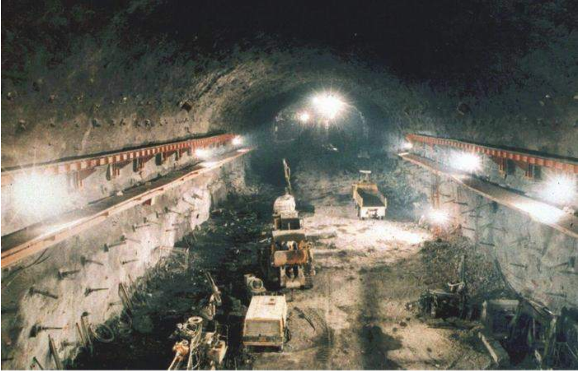
Figure 25: View of the Mingtan cavern from the platform of a temporary construction crane supported on rails bolted to the cavern walls.
