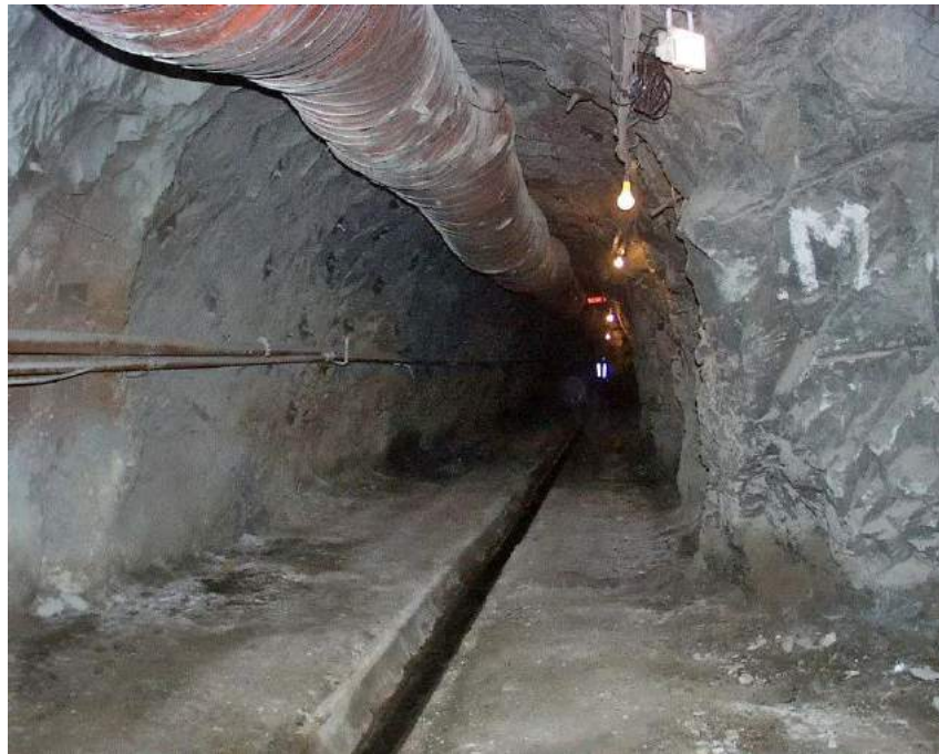
Figure 10: Appearance of the drainage tunnel in fair quality granodiorite in which no permanent support was required. Spot bolts and shotcrete were installed for safety in jointed areas. The concrete lined drainage channel is shown in the centre of the tunnel floor.
