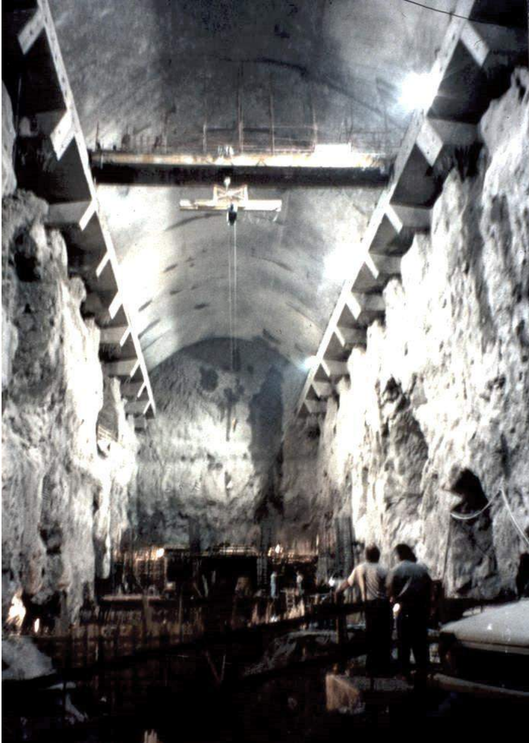
Figure 29: Crane beams rockbolted to the walls of the power cavern of the Thissavros hydroelectric project in Greece. These rails provided support for the temporary construction crane shown in the photograph. The stubs projecting from the bottom of the beams were later attached to concrete columns that provided support for the main crane.
