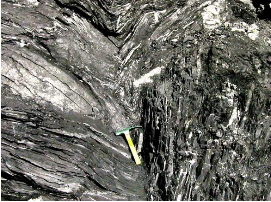
Figure 3: Tectonically deformed and sheared graphitic phyllite in the face of the Yacambú-Quibor tunnel at a depth of 1200 m below surface.
