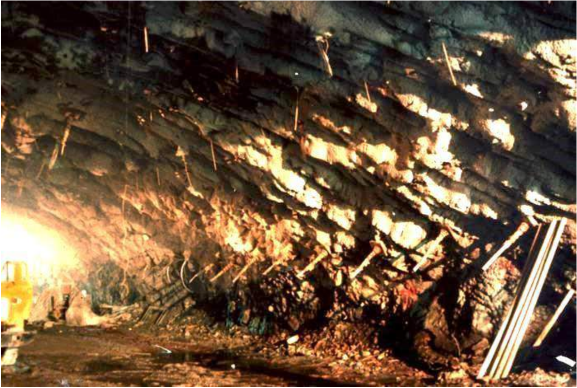
Figure 18: Blast damage in the first section of the cavern arch to be excavated.
