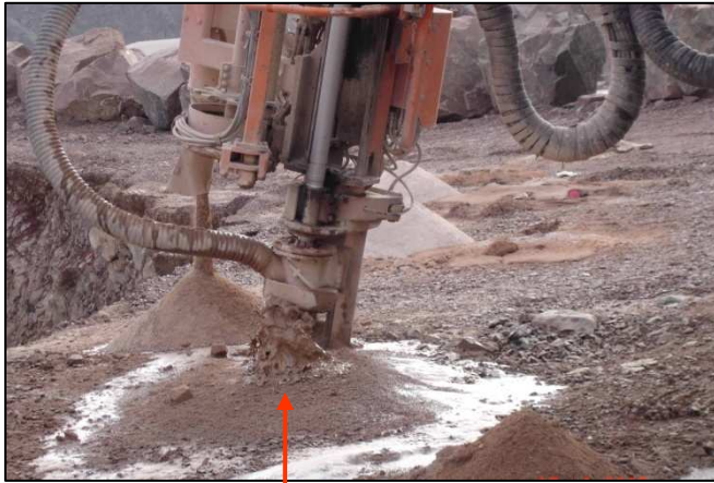
Burst of inhole water
