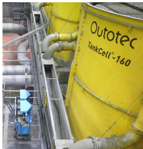
Figure 4.5: Location of pilot cells (lower left corner) next to industrial flotation cells.
